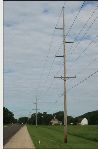
69-kV/115-kV transmission structure with distribution underbuild
