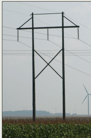
230-kV/345-kV H-frame transmission structure
